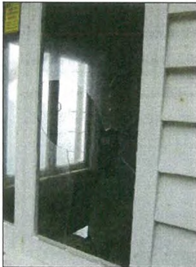
Photograph 17: Broken window to be repaired
