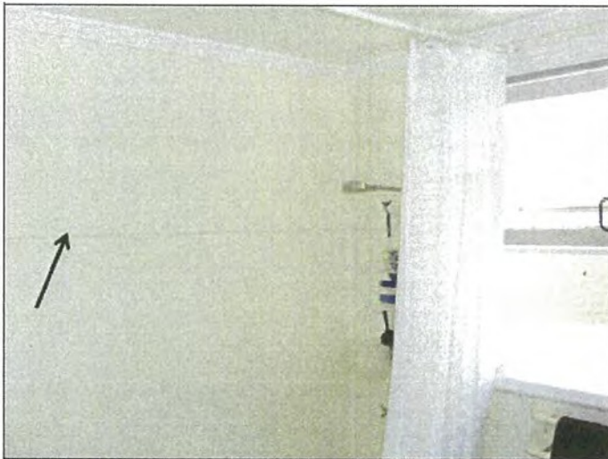
Photo S-7504: Bathroom, wall cladding in bath / shower area only Photo S-7508B: Bathroom, flat cover strips
