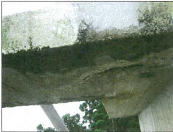
Photograph 21: Spalled concrete to underside of viewing platform
