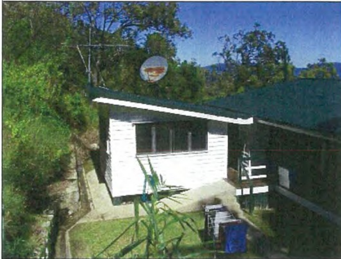
Photo S-7521: Roof sheets on House 2, Office section Photo S-7522: Edge capping on Office section
