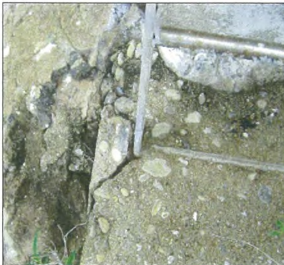
Photograph 24: Local concrete spalling at ladder support leg
