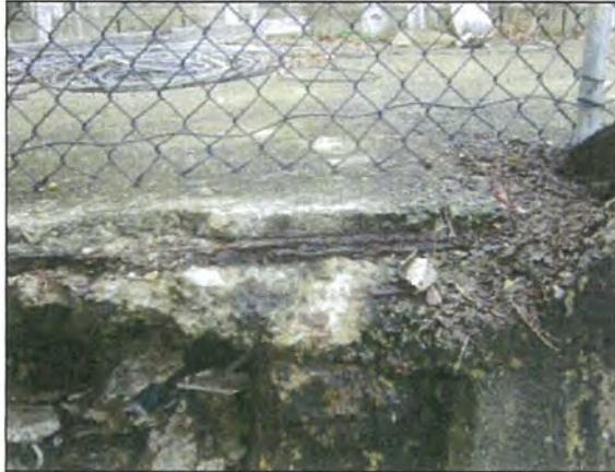
Photograph 7: Exposed reinforcement to slab edge
