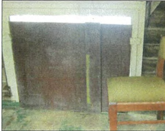
Photograph 18: Plywood infill panel to be replaced
