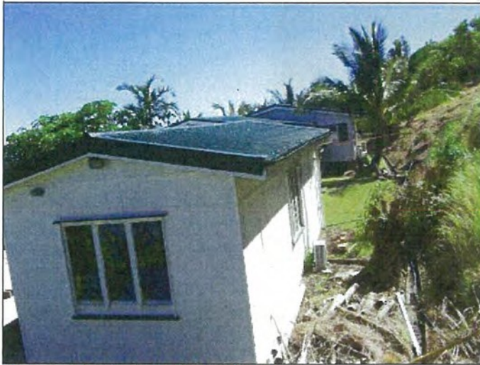
Photo S-7497C: Workshop Shed, roof cladding Photo S-7498D: Edge capping Photo S-7507C: Ridge capping
