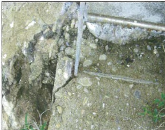
Photograph 11: Concrete spalling and corrosion of access ladder
