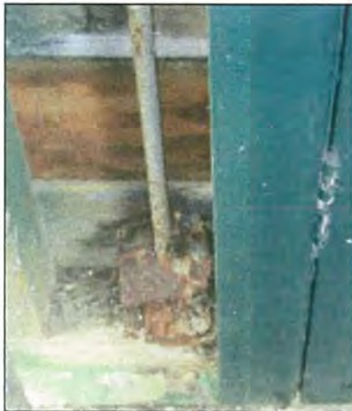
Photograph 20: Typical corroded base tie-down connection
