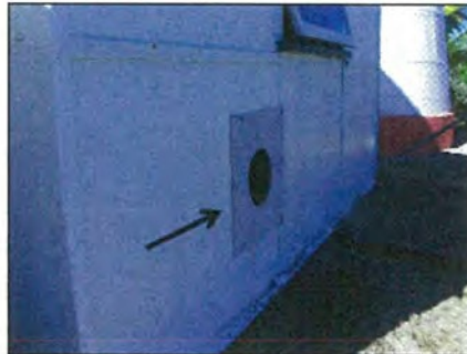
Photo: Gen. Shed, external South wall, unpainted patch panel is non-asbestos material (tested)
