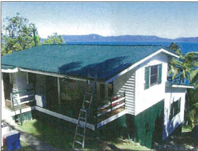
Photo S-7521: Roof sheets on House 2, House section Photo S-7522: Edge capping on roof Photo S-7507E: Ridge capping on roof
