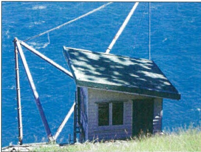
Photo S-7516: Winch House, edge capping on roof Photo S-7517: Roof sheets
