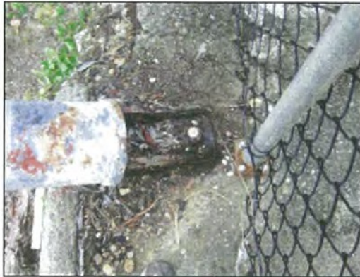
Photograph 9: Corrosion and debris around upper strut arm connection
