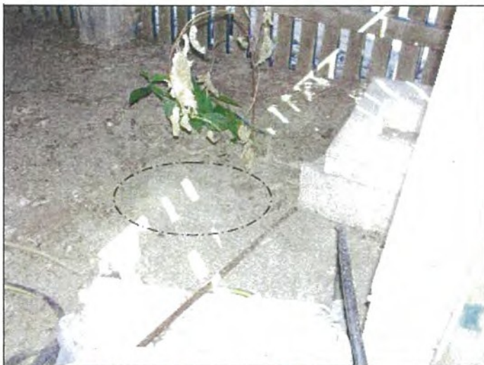
Photo S-7506: Debris in soil under House 1, Northern end
