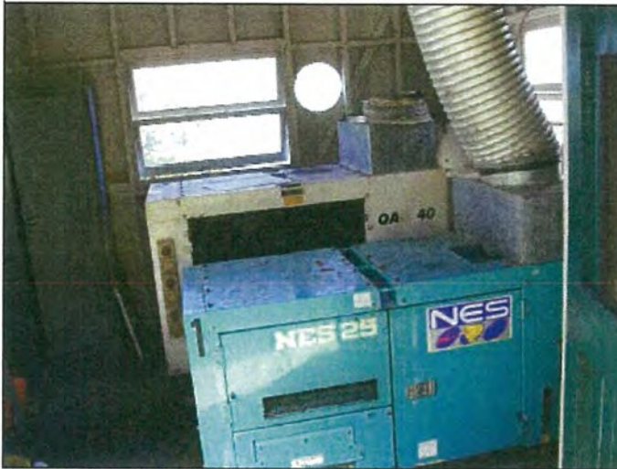
Photo: Suspect gaskets installed to generator motors
