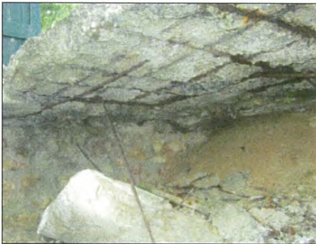
Photograph 6: Extensive corrosion and delamination of concrete slab
