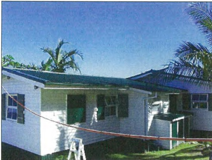
Photo S-7499: Roof cladding Photo S-7498B: Edge capping on roof Photo S-7507B: Ridge capping on roof
