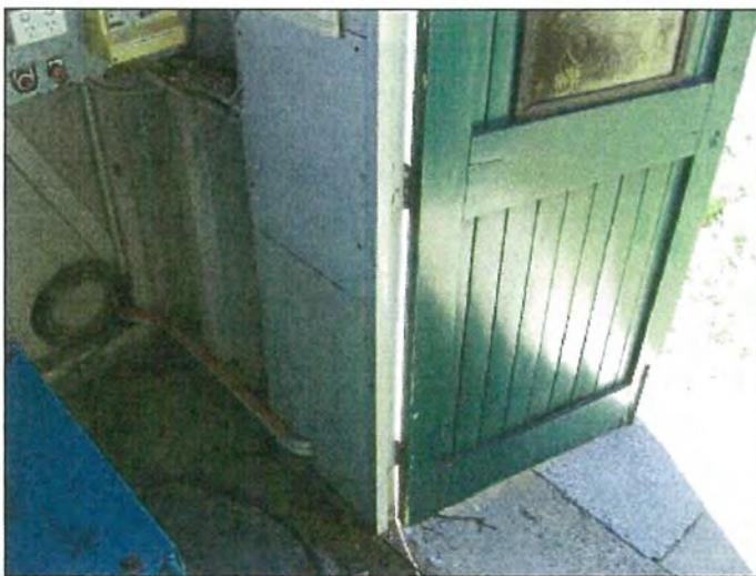
Photo S-7511C: Two (2) small wall panels at right upon entry to Gen. Shed
