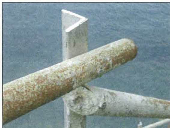
Photograph 12: Handrail with dissimilar metals in contact
