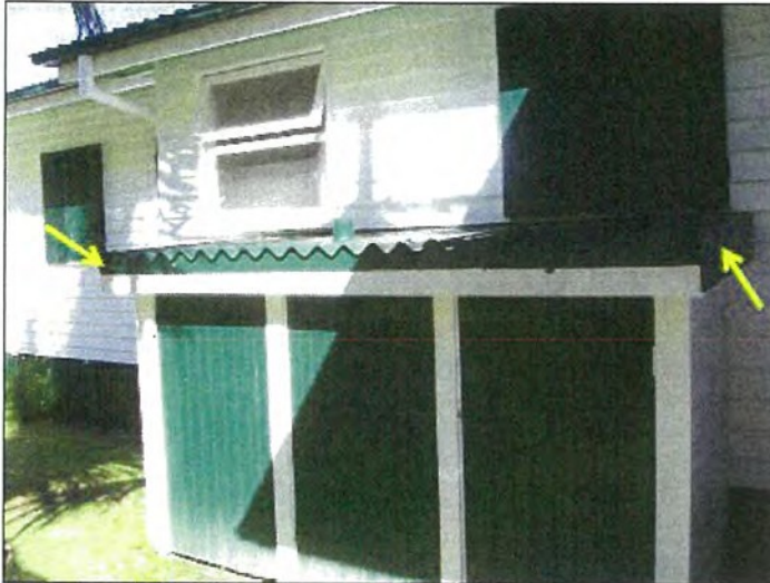
Photo S-7497A: House 1, roofing on Hot Water System box Photo S-7498A: Edge capping on roof of Hot Water System box
