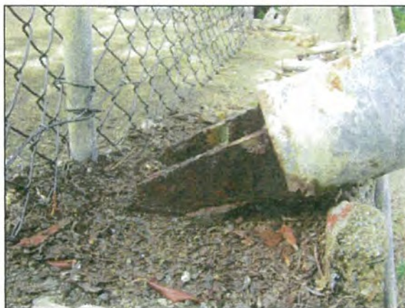
Photograph 22: Corroded base connection of strut to be repaired
