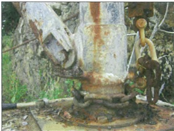
Photograph 8: Corrosion to central base connection
