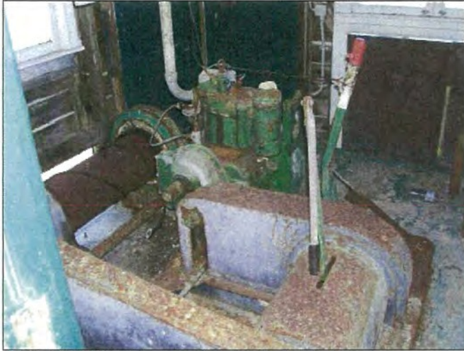
Photo: Winch House Suspect gaskets & brakes on winch motor
