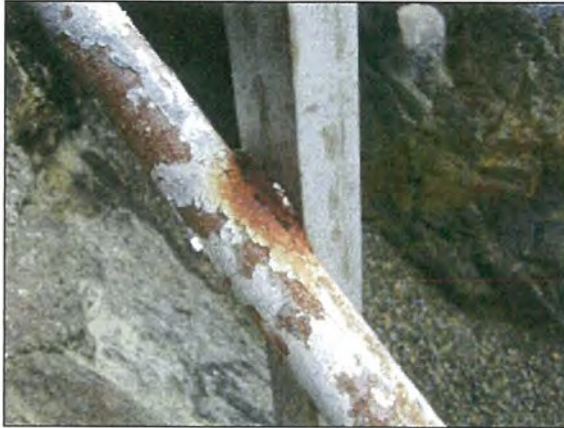
Photograph 13: Handrail with dissimilar metals in contact
